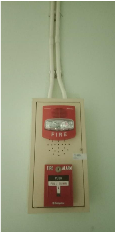
Current Manual Pull-Down Station x2/floor
